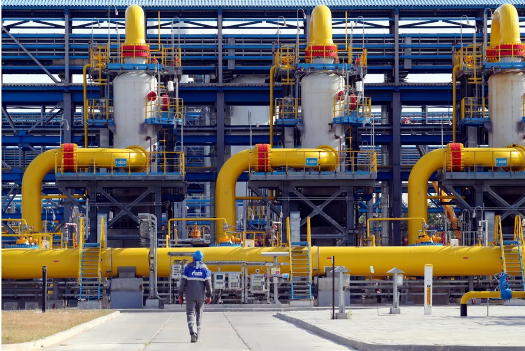
A worker at a compressor station for the Nord Stream 2 offshore natural gas pipeline, in Ust-Luga, Russia, in July 2021. Once operational, the Nord Stream 2 pipeline will supply gas from Russia to Germany. | Peter Kovalev/TASS via Getty Images
